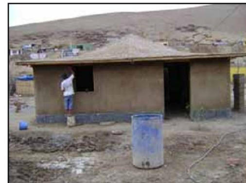
Figure 3.9 Mud plaster on an adobe house
